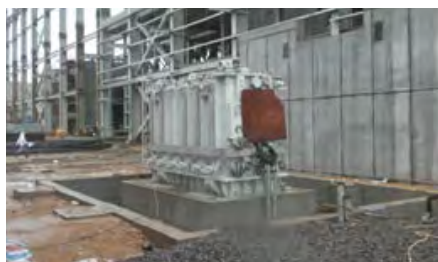
Main and standby transformers on their foundations
