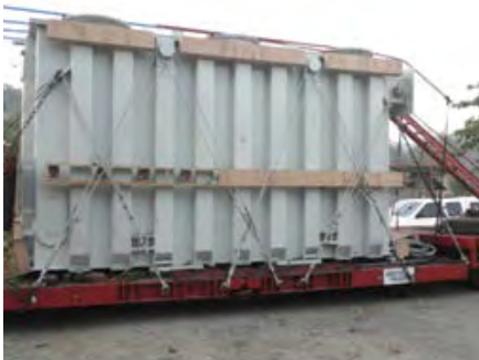
Transformers secured to SPMTs using Chains and Binders (T) and Wires and Turnbuckles (B)
